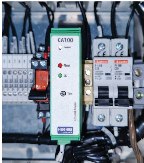
Installation in the motor drive cabinet
